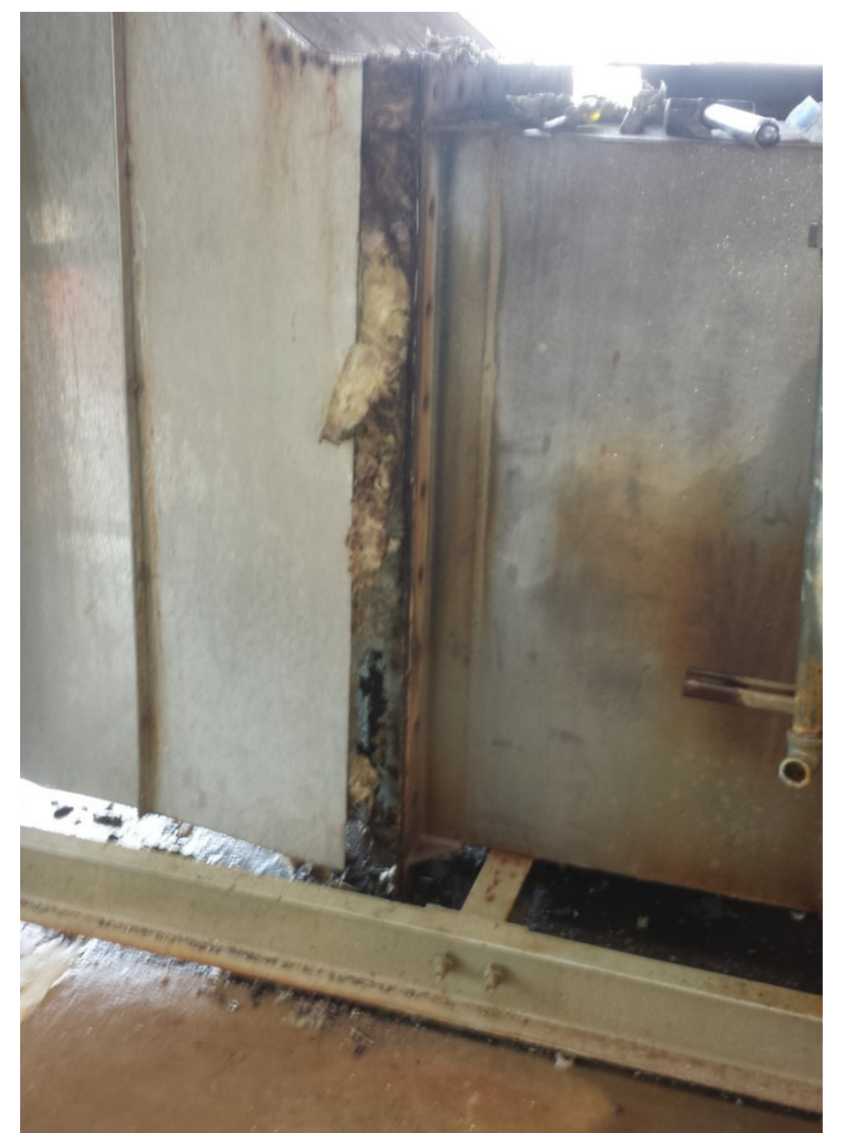
BEFORE: Connection at exhaust stack
